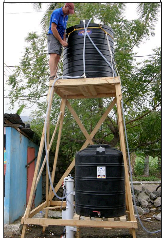
Erecting a water tower for the community child care centre in Petit Guinee
