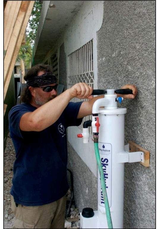
Safe water for the patients, staff and visitors in a hospital in Carrefour
