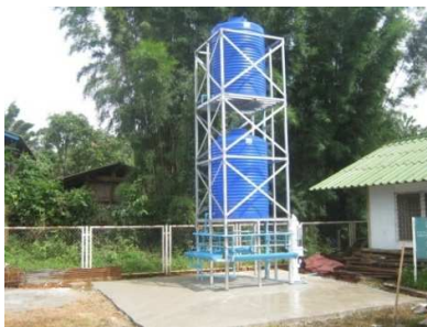
If well maintained, this water system tower can last for at least 10 years.
