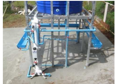
Front view of the water system
