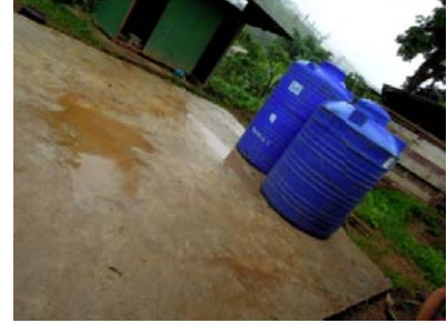
The community had laid the foundation with Childs Dream instructions before the team arrived!
