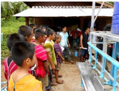
If well maintained, this SkyJuice water filtration system and tower can last for at least 10 years.
