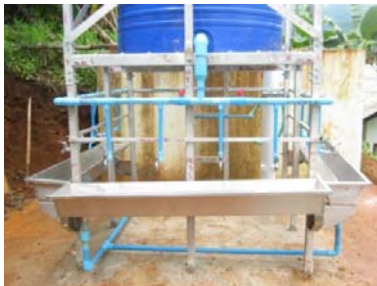
If well maintained, this water system tower can last for at least 10 years.
