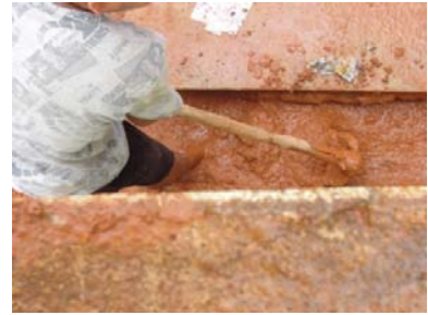
The drains had to be cleared of mud to install the pipes
